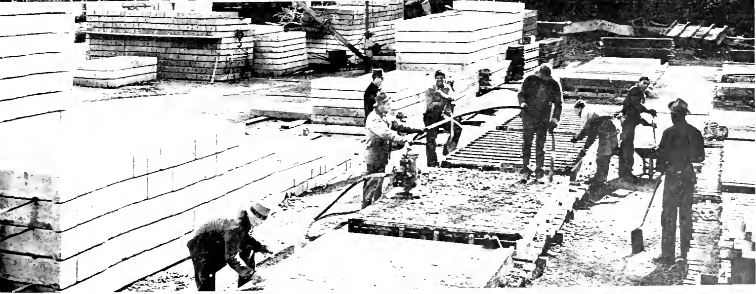
Precast cribbing protection on Trinity River. Below—Making 15,000 concrete crib members at camp between Junction City and Helena
